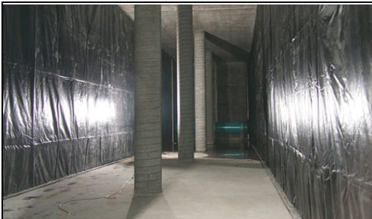
Figure 2: Typical fixed baffle curtain located inside a water treatment facility
